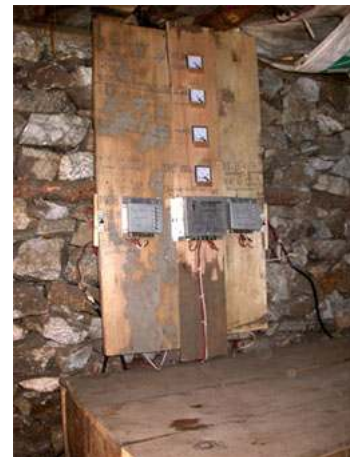
Picture 37: Charge- / discharge-controller, with separate load controller, inside the power house.
