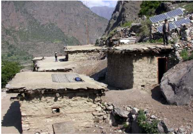
Picture 33: In the middle of the village of Chauganphaya the local people have provided the land to build the central solar PV system power house. From the power house all homes are connected via armored underground cable, buried at a depth of 50 – 80 cm.
