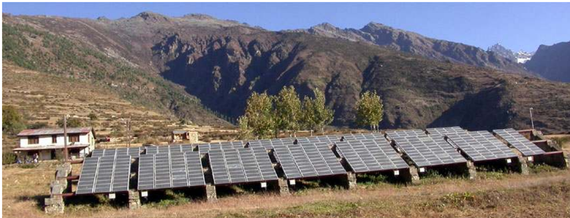
Picture 1 35 : Simikot Humla 50 kW R Solar PV System, after 16 years of operation
