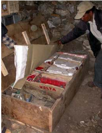
Picture 38: The battery bank well insulated in a locally made wooden box.
