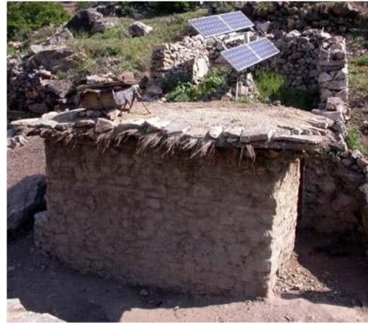
Picture 34: The local people built the power house with their own materials. It contains the battery bank, which provides up to 5 days power for all the lights during no-sun days, and a charge and load controller (pictures 37 & 38).
