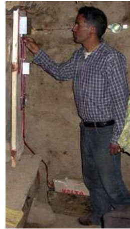
Picture 30: Checking the battery and charger
