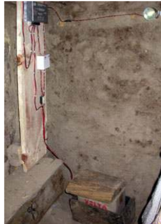
Picture 29: Cluster power house with charge controller and battery
