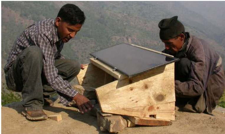
Picture 31: Project staff and user install the solar PV systems together, creating knowledge, skills and ownership
