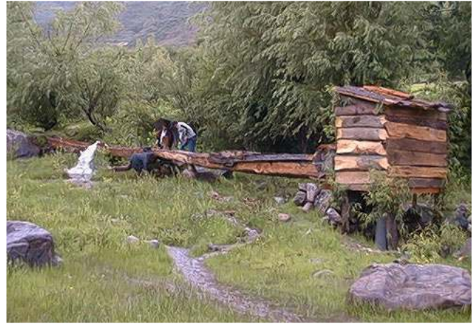
Picture 10: The power house, and the water canal of the Godhigau village 165 watt pico hydro power plant are built with local wood, with no cement which is prohibitive expensive.
