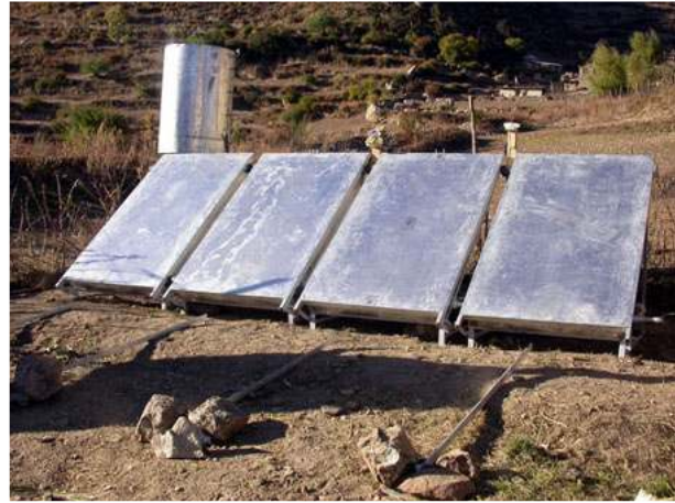
Picture 3: The High Altitude Thermo-Siphon SWH in closed, or after sunset, position. The insulation all around the absorbers and the hot water storage tank consists of 100 mm polyurethane foam. Four thermocouples on one absorber measure the water temperatures at different heights, and 4 thermocouples, installed at different heights, measure the hot water storage tank temperature and stratification. All data is recorded every minute for the first 5 months of field tests during the winter of 2005/6. Initial efficiency calculations showed values of 45% - 55%.
