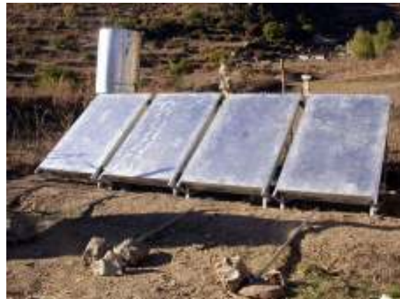
Figure 2-8 The HASWH in closed, freezing night position. Absorber boxes and hot water storage tank are insulated with 50mm and 100mm polyurethane foam respectively. Four thermocouples on one absorber and four in the hot water tank, each at different heights, record the different water temperatures. All data is recorded with a dataTaker DT605.
