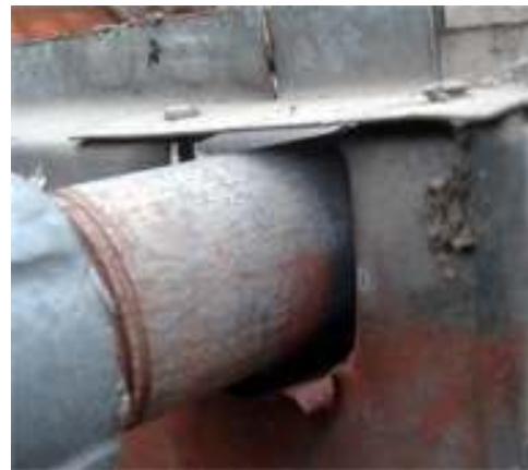
Figure 2-3 SWHs are poorly manufactured, with cheap materials and thus high unnecessary heat losses occur.
