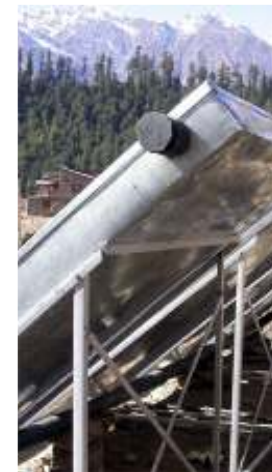
Figure 2-14 In order to maximise the winter hot water generation, the absorbers are at 40° South installed at a latitude of 30° North.
