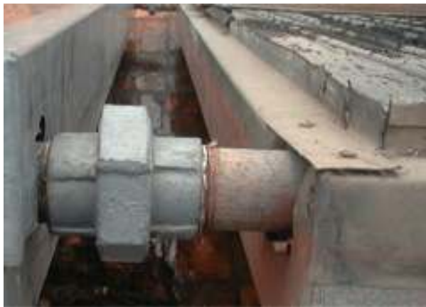
Figure 2-2 SWH without pipe insulation, insufficient absorber insulation, and poor absorber blackboard paint.
