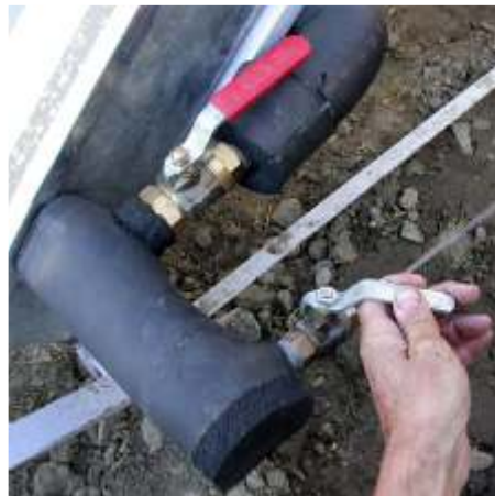
Figure 2-13 Valves at the bottom of the absorber unit. Once the hot water storage tank inlet valve is closed and the top drain valve is opened, the bottom valve is opened and the absorber water circuit is emptied. In this way only air remains inside the absorber pipes.
