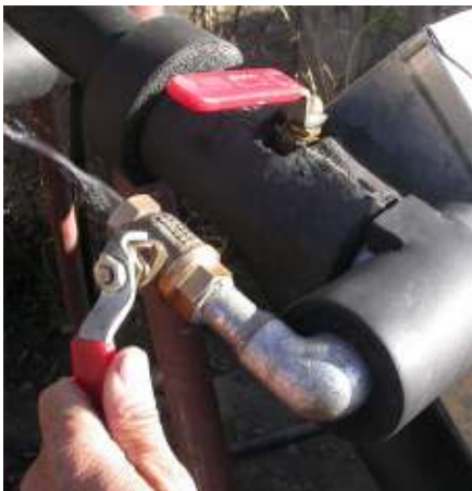
Figure 2-12 The drain and the hot water storage tank inlet closing valves at the top of the absorber unit. They isolate the storage tank from the absorber unit as part of the freeze protection during the cold, 5-6 freezing winter month, nights.
