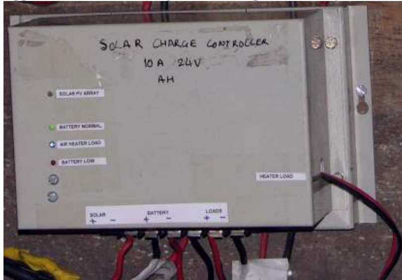
Appendix 3: Photo of Charge Controller (photo courtesy of Alex Zahnd)
